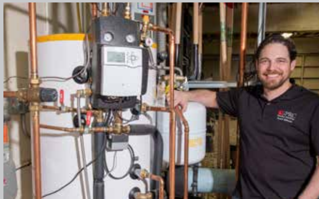
Plumbing Instructor Brett Dillman with the solar powered hot water boiler students use in the lab.
